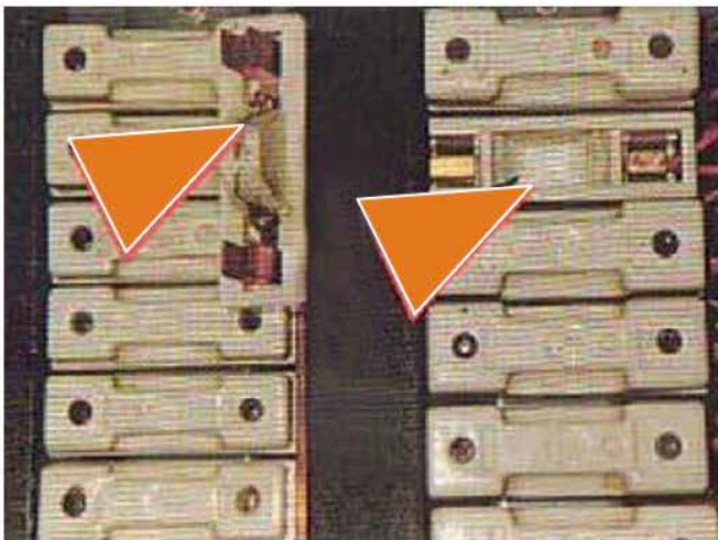
Asbestos Rope (electrical fuse board)
