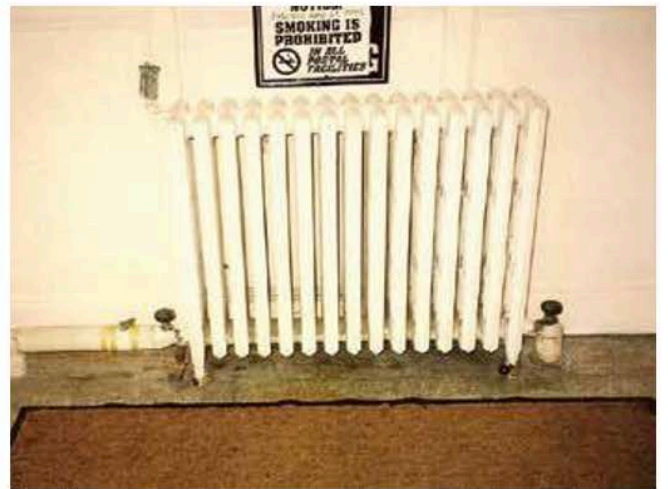
Radiator (insulation on piping and valves)
