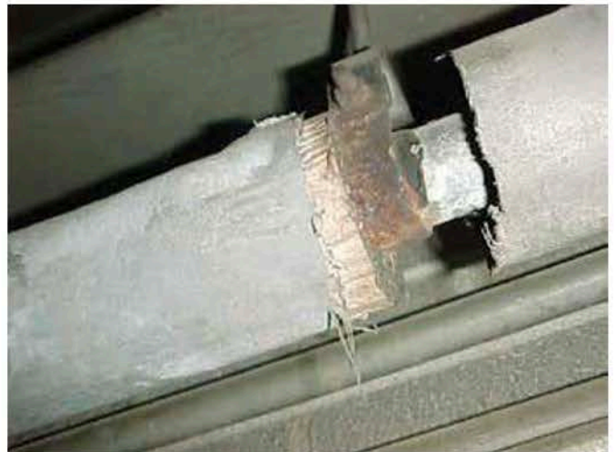
Pipe Insulation (damaged)
