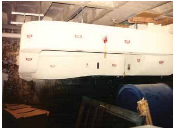
Heating and Cooling Duct Insulation (HVAC)
