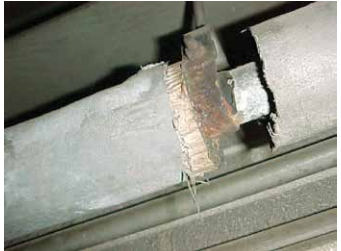
Pipe Insulation (damaged)
