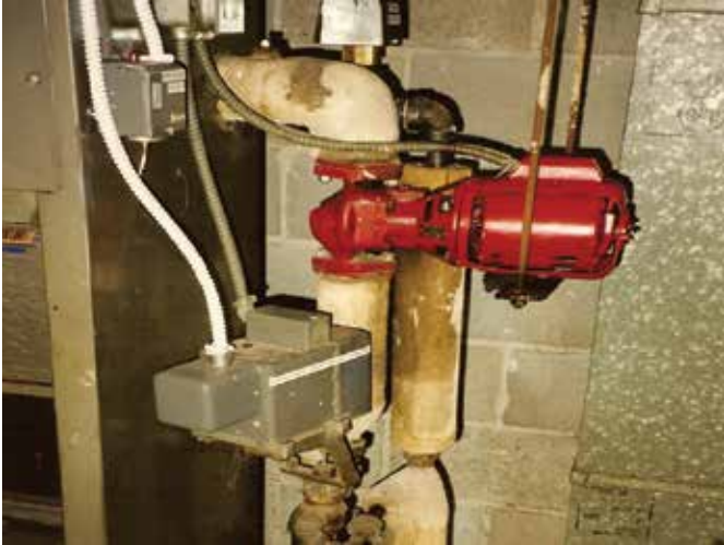
Fire Sprinkler Pump Piping Insulation
