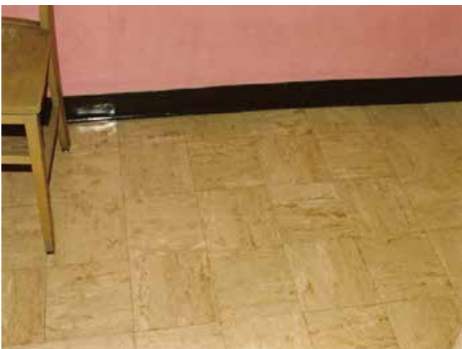
Vinyl Floor Tiles and Cove Base (most 9" x 9" and 12" x 12" floor tiles)
