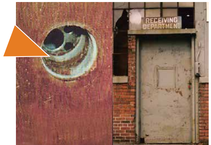
Fire Door (insulation inside door)
