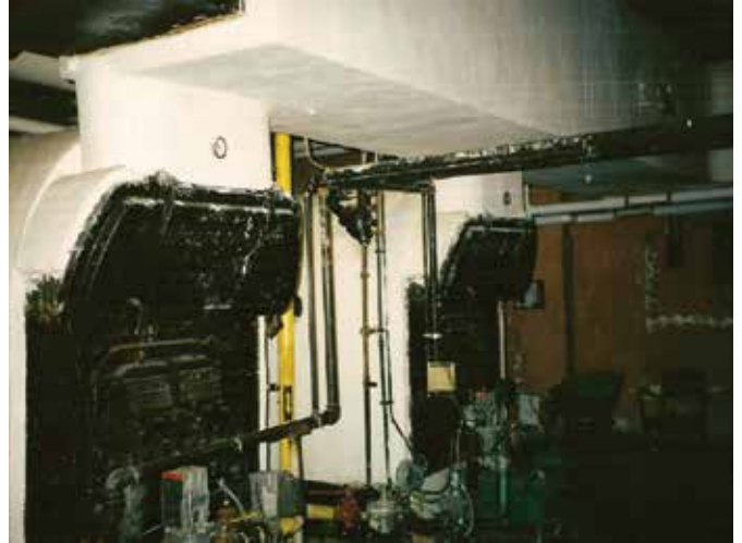
Boiler and Pipe Insulation
