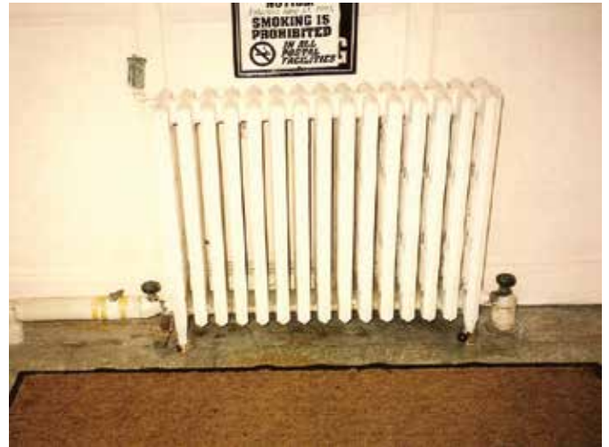
Radiator (insulation on piping and valves)
