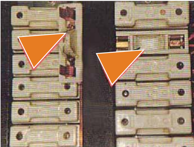
Asbestos Rope (electrical fuse board)
