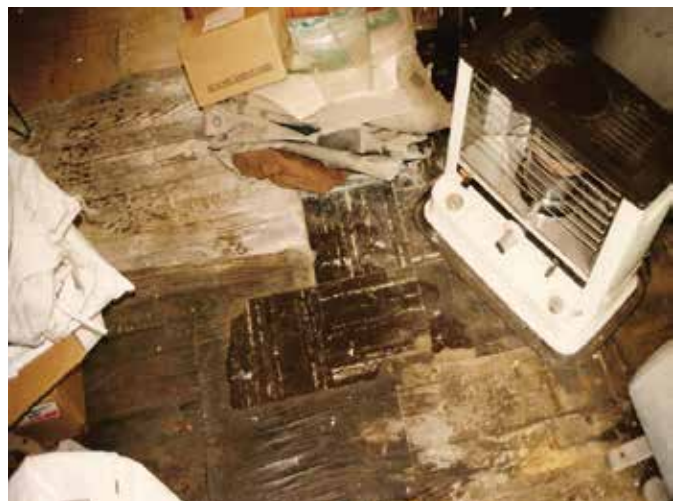
Vinyl Floor Tiles and Adhesive Mastic (on wood floor, damaged 9" X 9" tiles)
